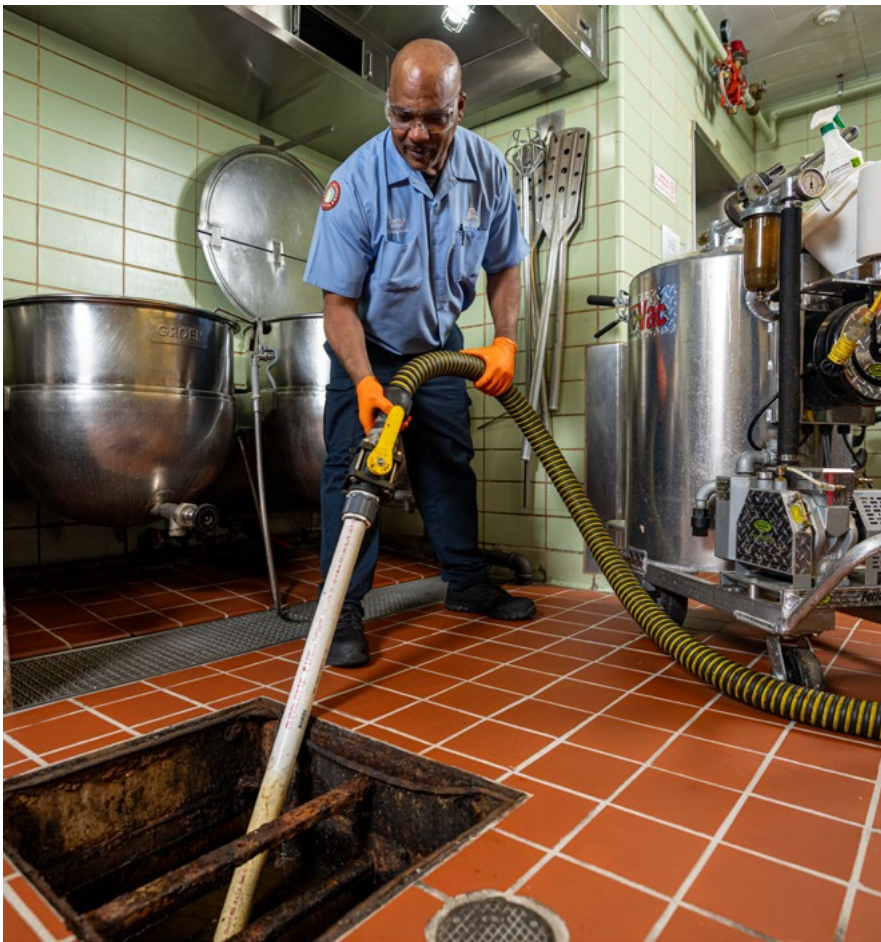
Watts vacuums kitchen waste from an underfloor pit.
