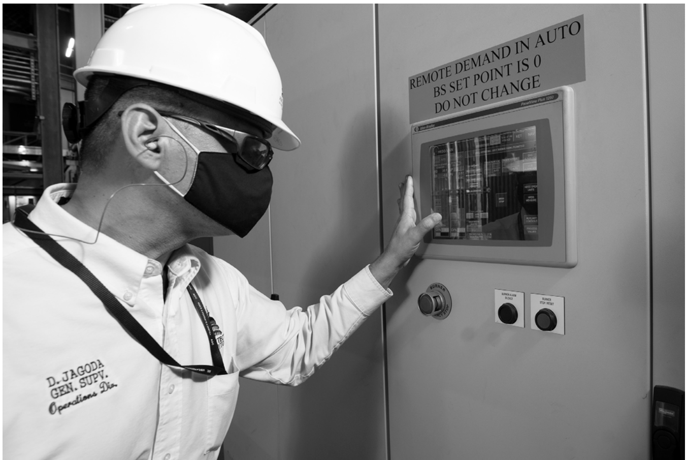
Jagoda at one of the cogeneration system control panels
