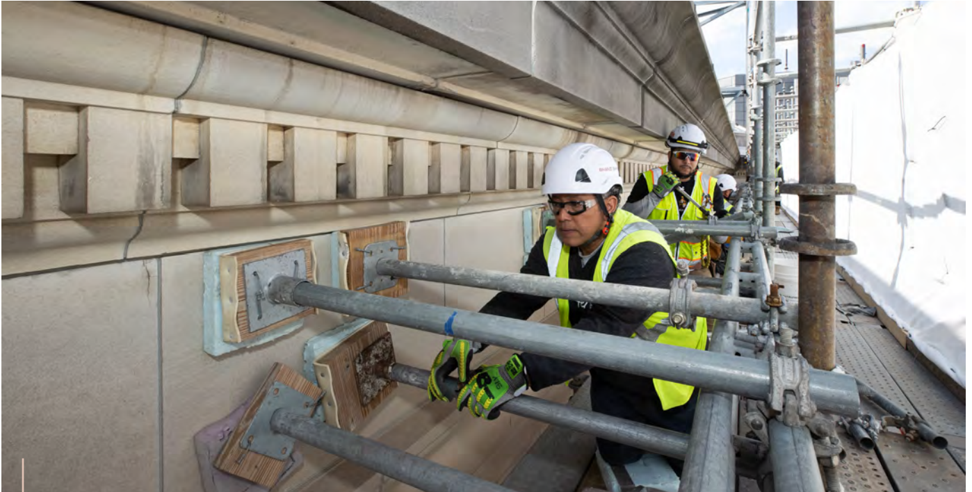
The Cannon Renewal project continued in FY 2023. Scaffolding allowed access to repair the stone exterior.
