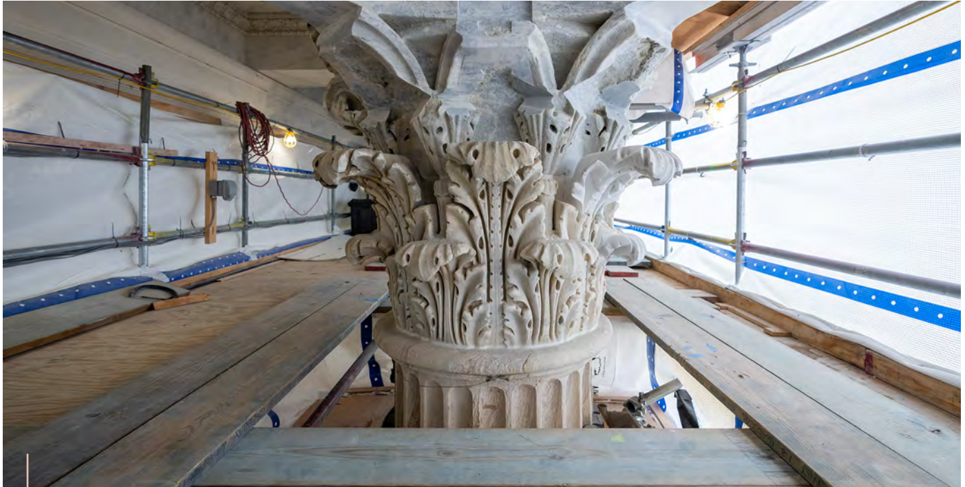
Column capitals were repaired during FY 2023 as part of the U.S. Capitol Exterior Stone and Metal Preservation Project.
