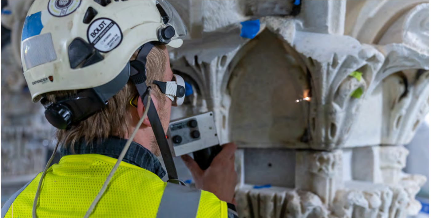
Dutchman repairs were completed on numerous column capitals and other stonework throughout the Capitol campus in FY 2023.
