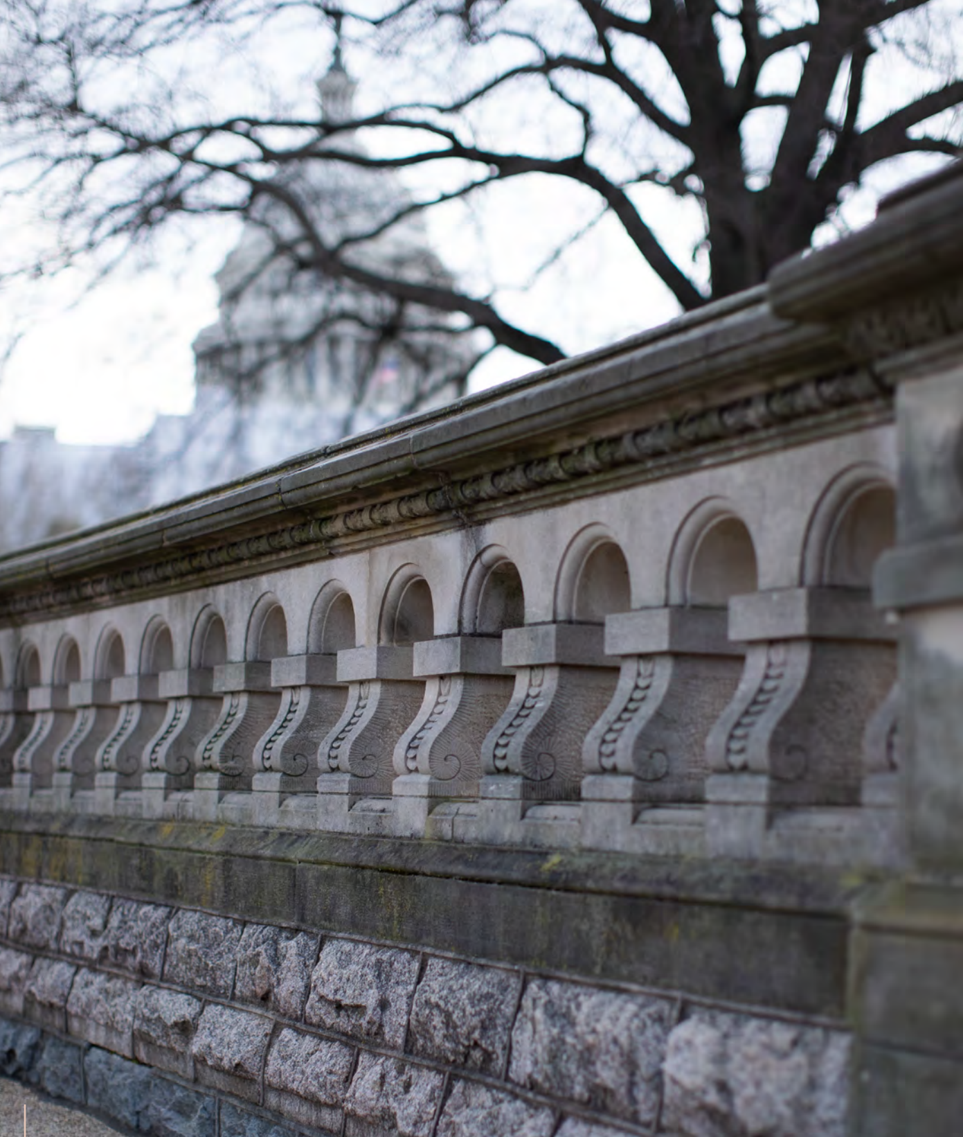
The Olmsted Terrace walls span nearly 1,600 linear feet and reach a height of approximately 20 feet.
