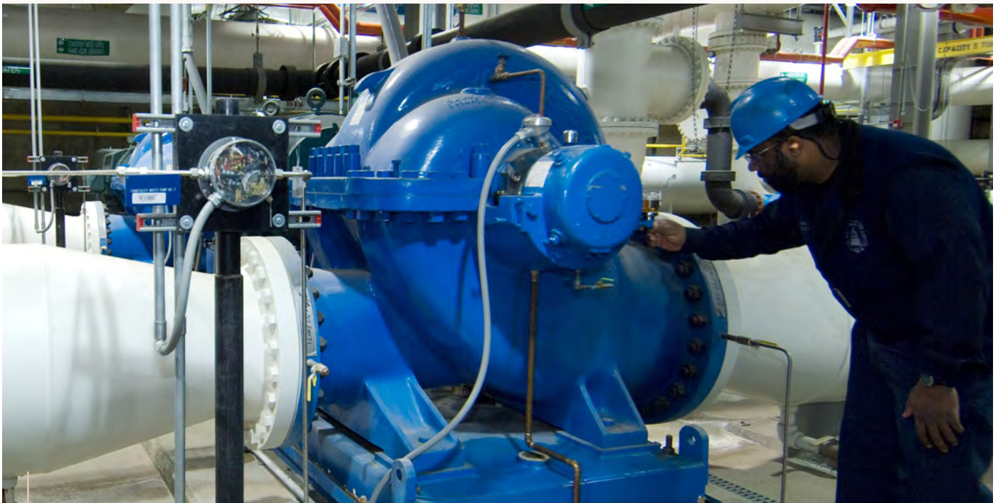
The Capitol Power Plant provides steam and cooled water to heat and cool the buildings across the Capitol campus.
