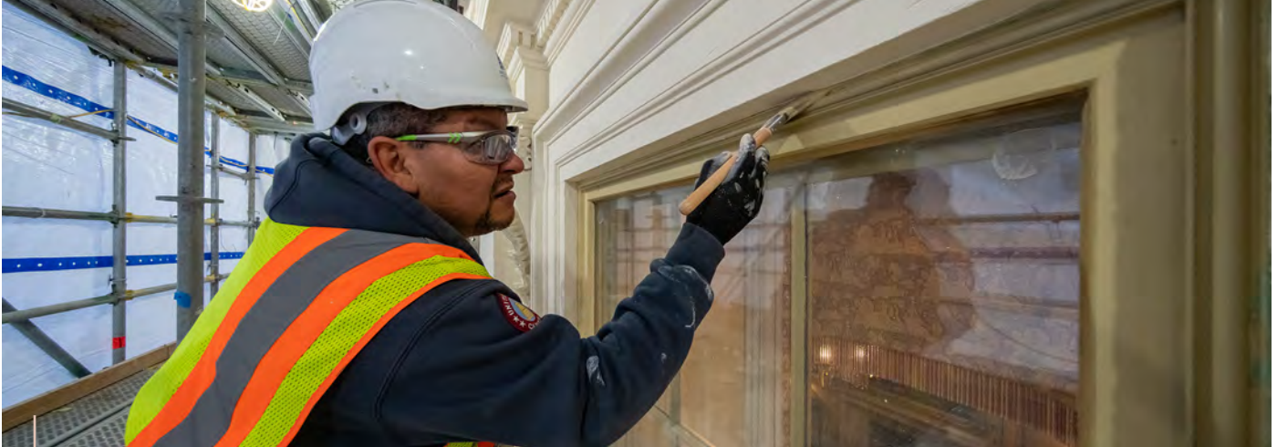
A craftsman repaints a window frame on the U.S. Capitol as part of Phase 3 of the U.S. Capitol Exterior Stone and Metal Preservation Project.
