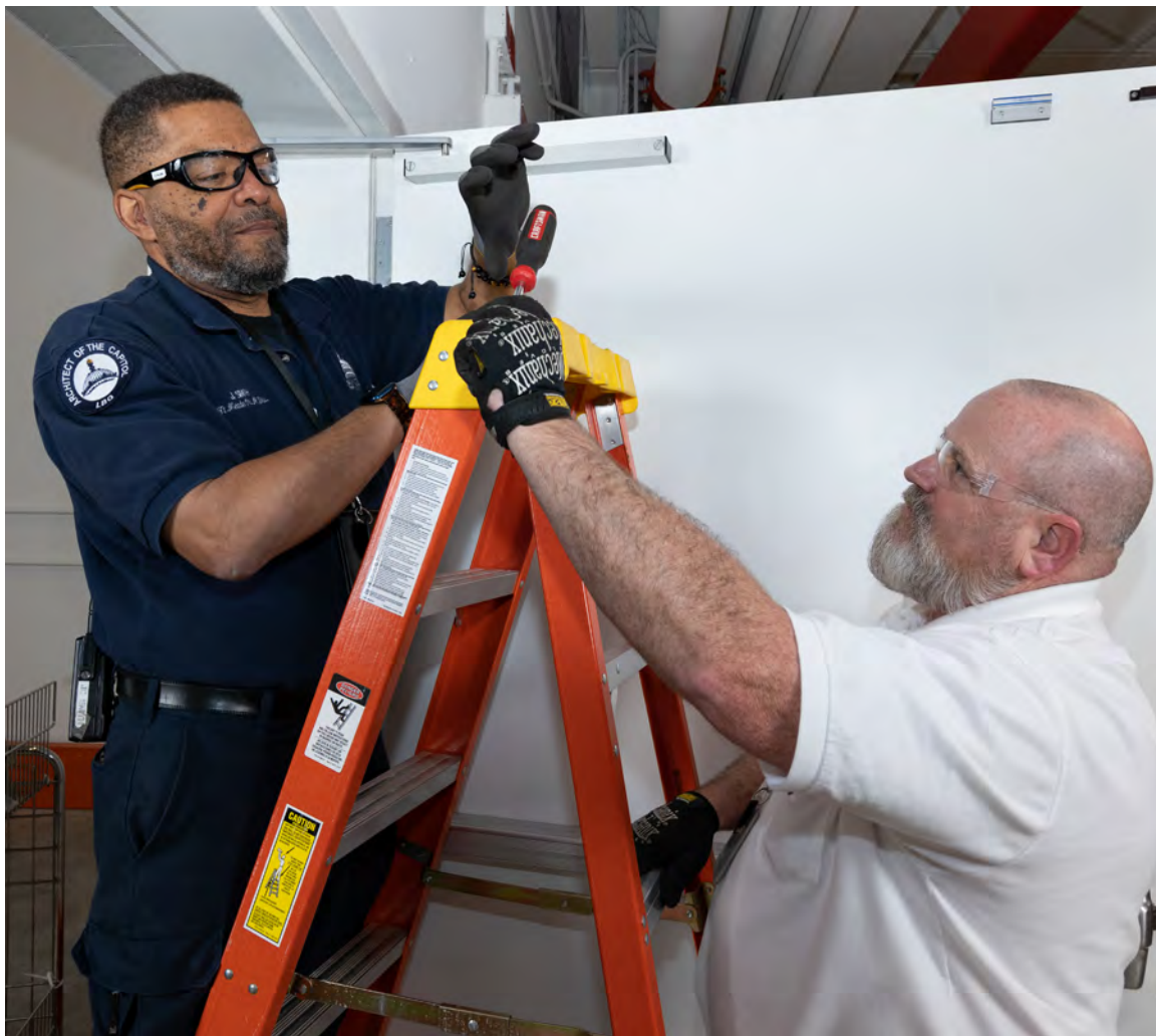
John Smith and Derrick Smith repair the automatic door closer in Module 4.
