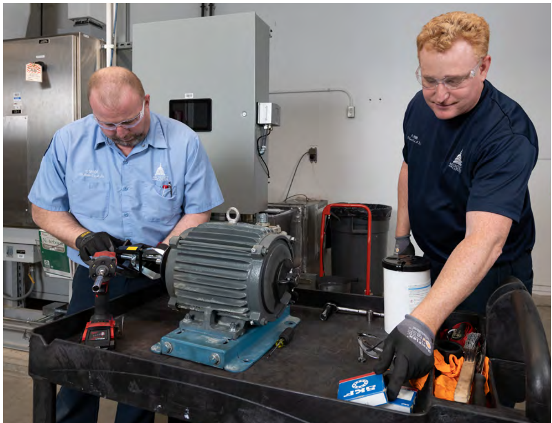
▼ Chris Saylor and Rick Webb service a fan motor for one of the cold storage rooms.
