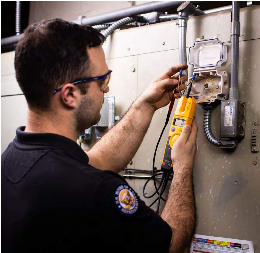
▼ A/C Equipment Mechanic Justin Zibragos tests temperature sensor function using an electrical tester.
