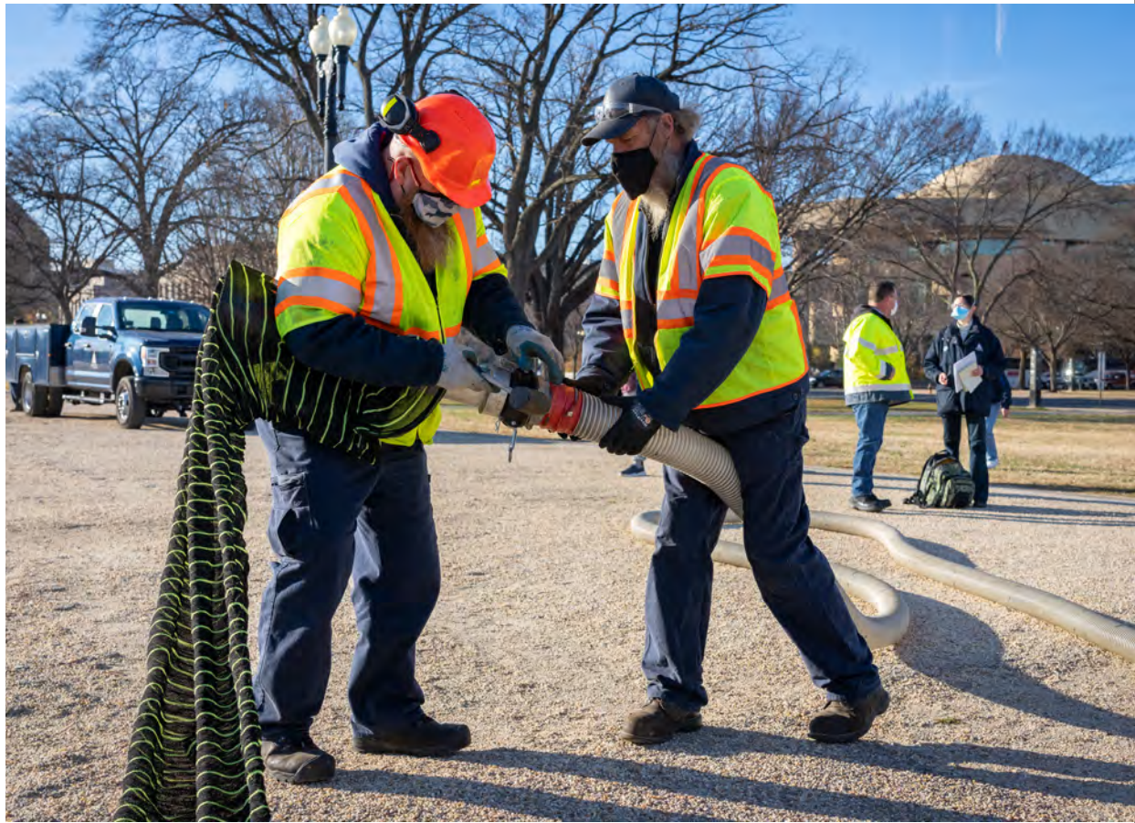
▼ Frank Bussler (left), Engineering Equipment Operator for Capitol Grounds, helps Richard Caselman, Heavy Mobile Equipment Mechanic Assistant Supervisor for Capitol Grounds, attach silt sock material to the end of a hose during a demonstration of the jurisdiction's new mulch blower.
