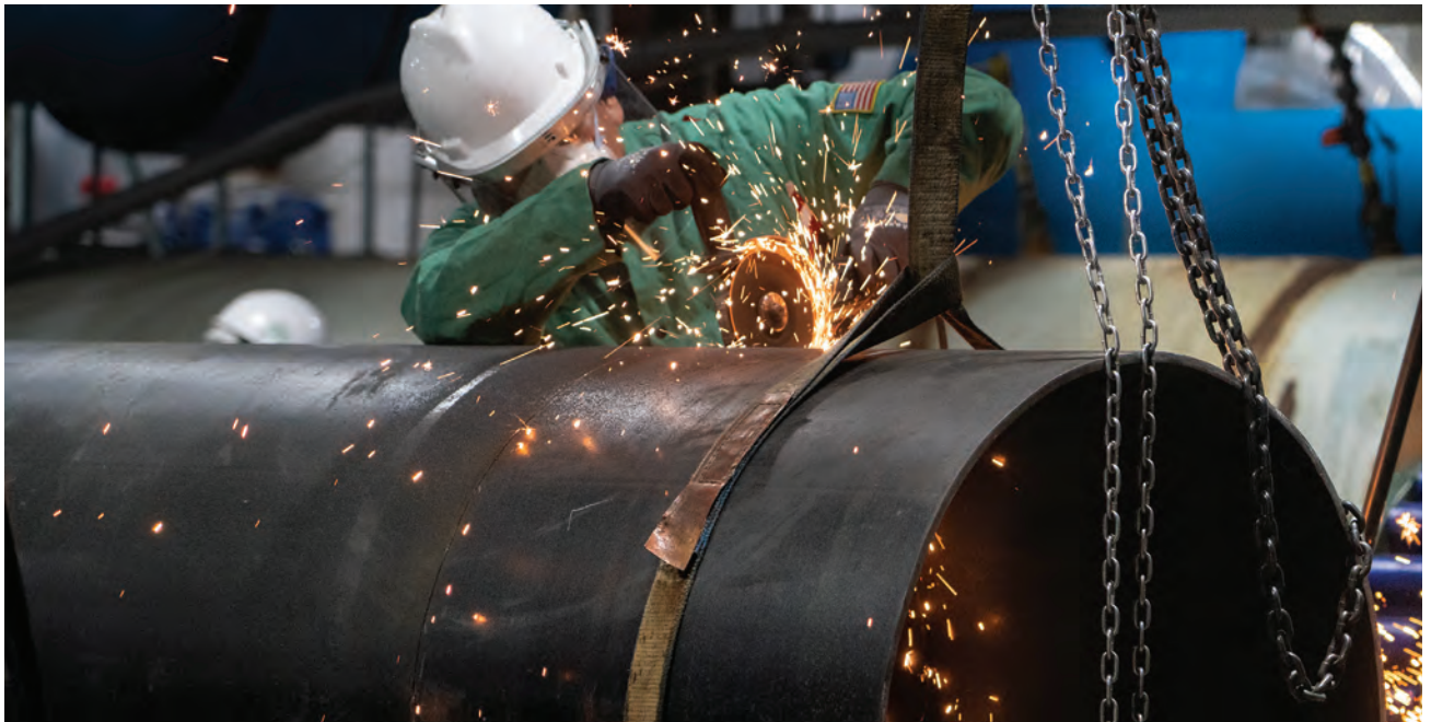
Above Major energy and sustainability infrastructure improvements at the AOC have been funded through public-private partnerships, including a utility energy service contract to fund the Capitol Power Plant’s cogeneration system.
