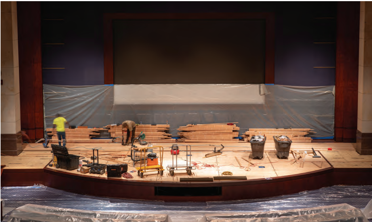
Above During October 2019, the AOC installed new stage flooring in the U.S. Capitol Visitor Center's Congressional Auditorium. During the COVID-19 pandemic, the Congressional Auditorium was used to support congressional hearings with proper social distancing requirements.
