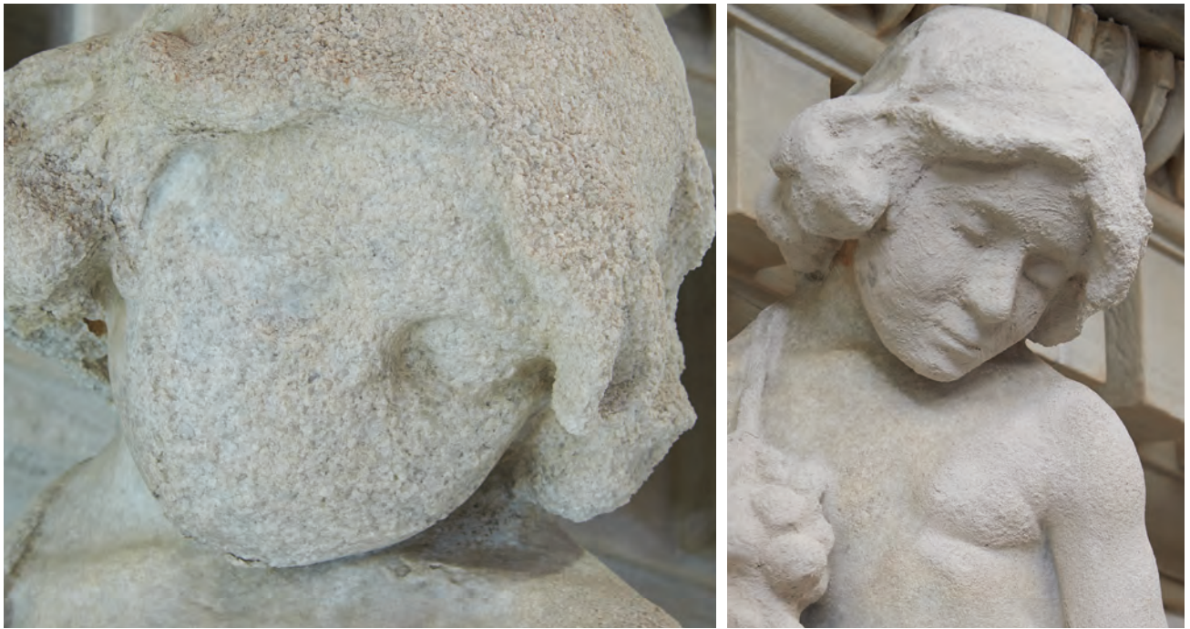
Above A detail on the U.S. Capitol’s House pediment before (left) and after restoration (right). Phase 2 of the U.S. Capitol Building Exterior Stone and Metal Preservation Project included the replacement of missing or irreparable stonework. This project is part of deferred maintenance and capital renewal backlog, the agency’s most critical management challenge.
