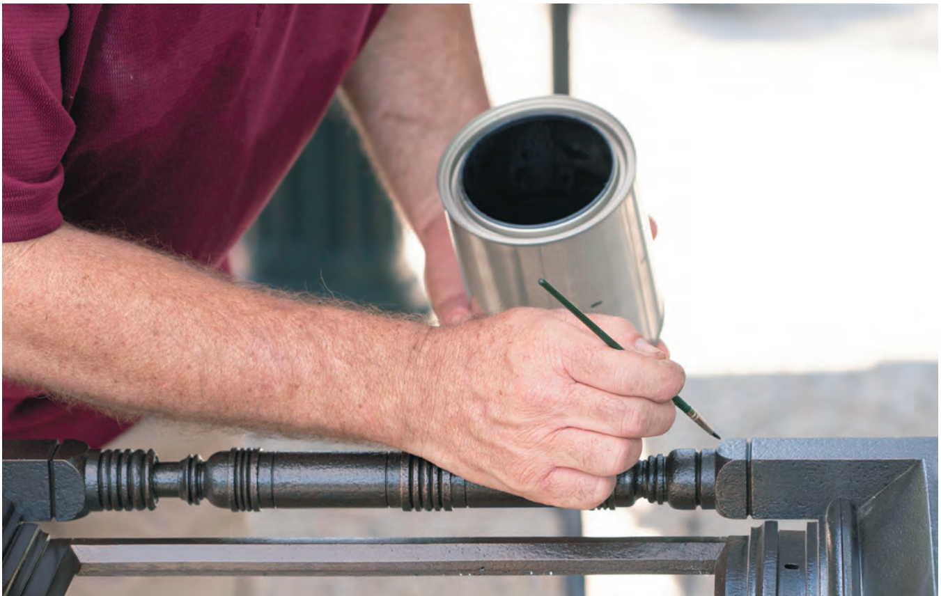
Touching up protective lacquer on the bronze framing of a lantern before it was reinstalled on its stone pier.
