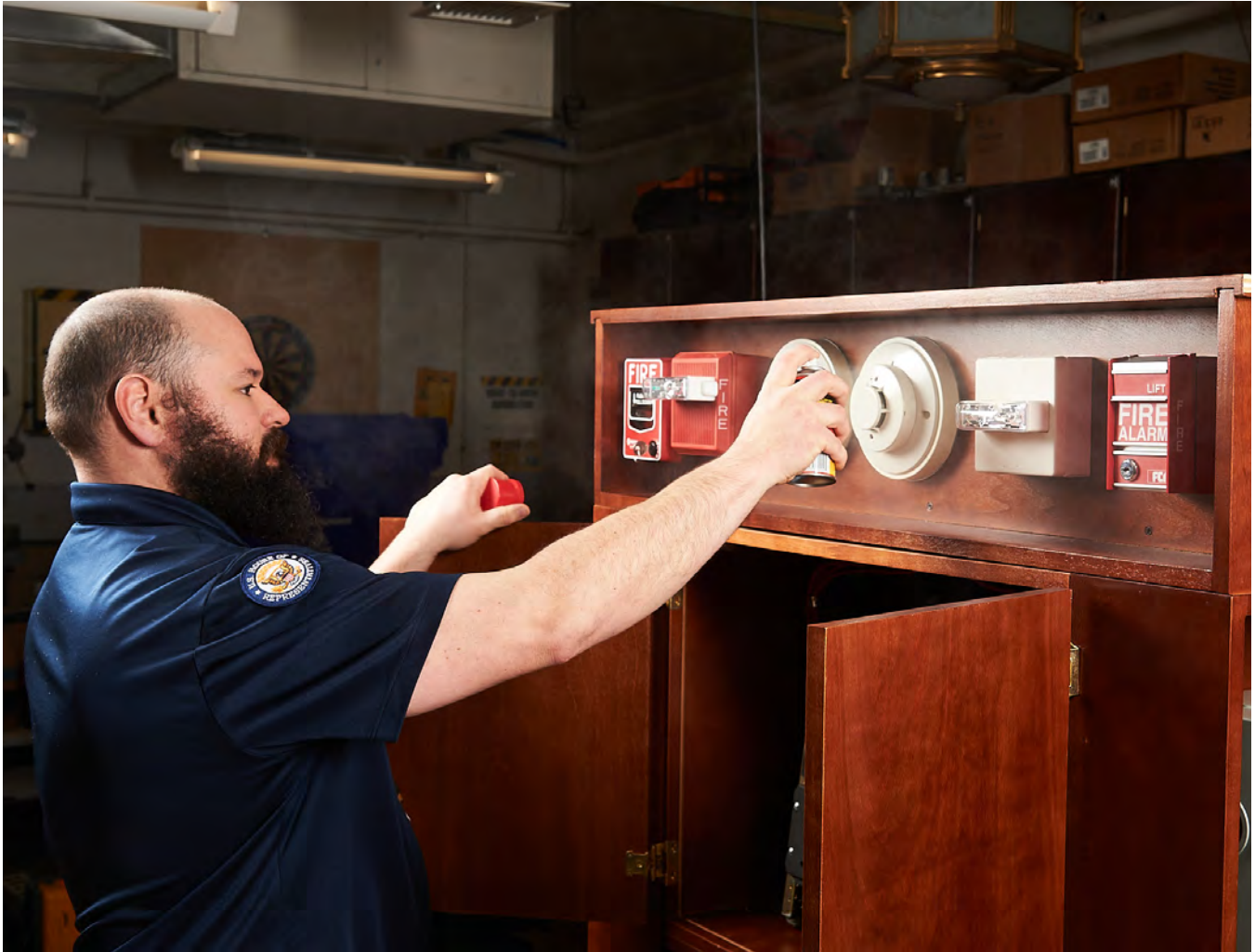
Greenwell sprays a can of smoke on one of the fire alarms to set it off.
