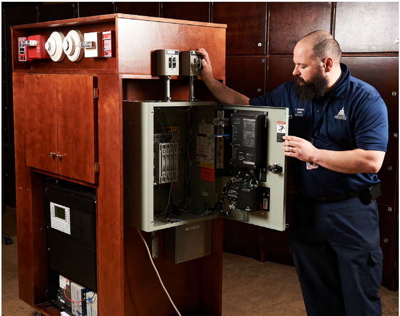
Greenwell operates the automatic transfer switch.
