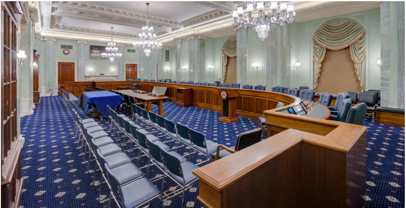
Top left: Quincy Biggs, painting worker with the Senate Painting Branch, paints the anteroom's new wall, which was added to conceal upgraded lighting controls and audiovisual equipment.
