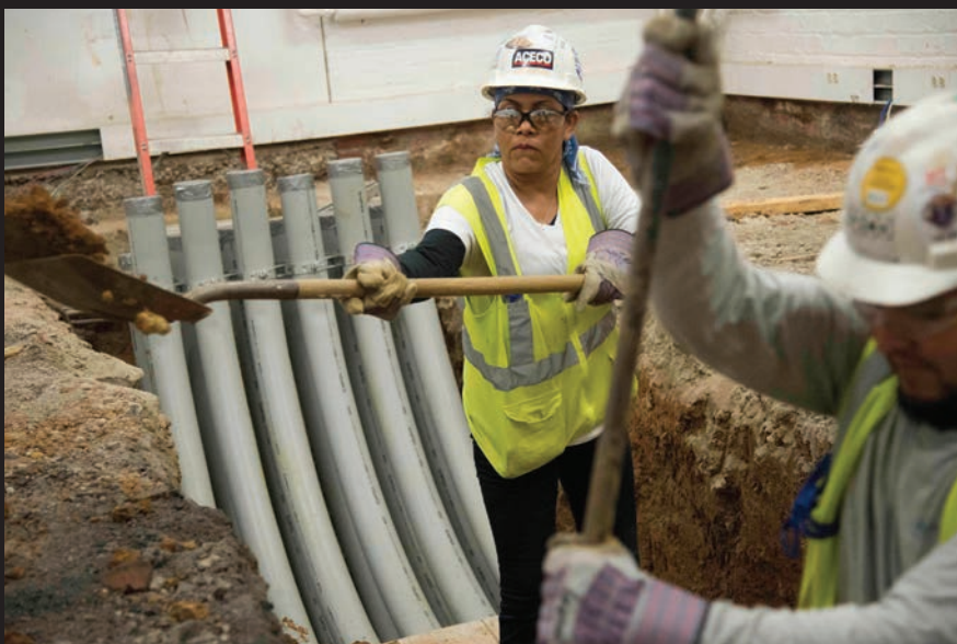
In March, the Cannon's east basement corridor was closed for five months to allow crews to begin to excavate the area and install utility infrastructure that will support the new mechanical and electrical systems.
