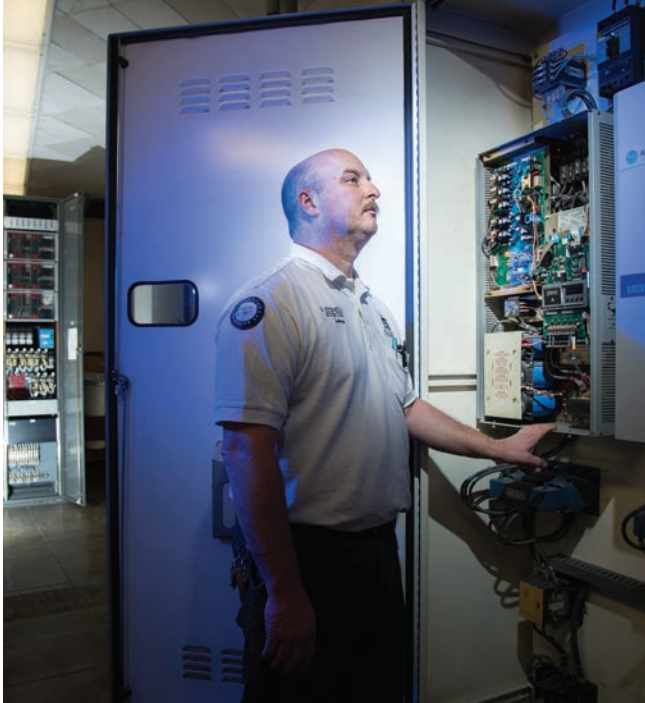
TOP: In a nearby mechanical room, Eric Fitzpatrick, who has 21 years of experience with the Senate Subway Branch, looks over the frequency drives for the subway system to the Hart and Dirksen Buildings. These drives power the fully-automated linear induction motors in the tracks, which make the cars go.
