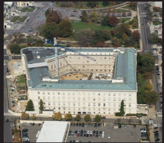
This aerial photograph, taken in November, provided a bird's-eye view of the Cannon Building and captured the 208-foot crane in action. Photo by Chuck Badal
