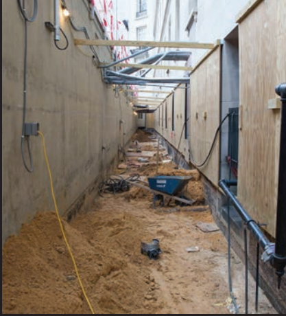
The perimeter of the Cannon courtyard was excavated an additional three feet to accommodate a future utility tunnel, as shown in this photo from June. These utilities will service the entire building and allow crews to isolate one side of the building at a time during future phases without interrupting service.
