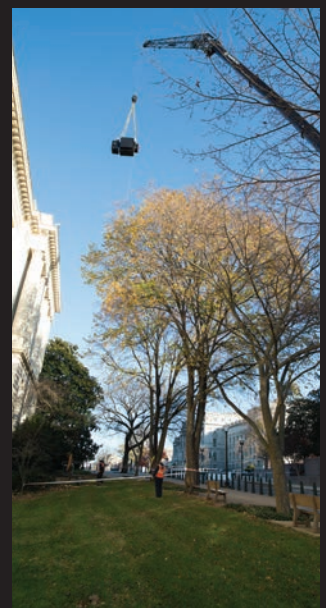
In December, crews replaced one of nine transformers with the help of a temporary crane set up on First Street, SE.
