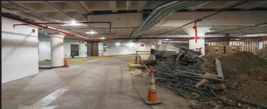
In January, the west side of the Cannon garage was closed to install the tower crane, utility piping, mechanical and electrical rooms, and to perform select demolition in the Cannon courtyard.
