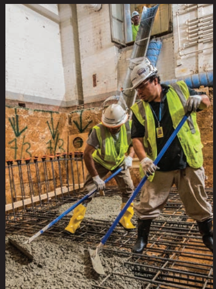
In May, workers placed concrete in one of the rooms adjacent to the east basement corridor.
