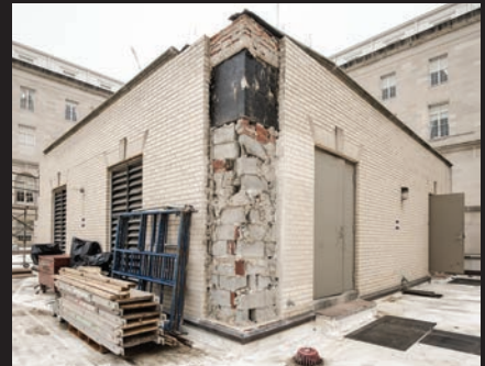
In April, demolition of the mechanical rooms and systems began in the Cannon courtyard. Crews were able to salvage historic limestone from these structures.
