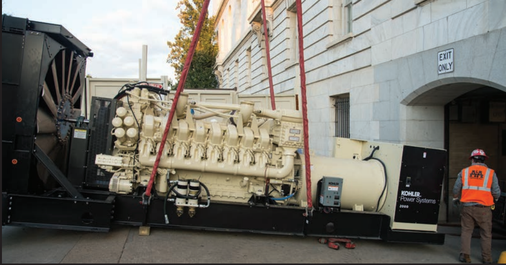
A new emergency generator was delivered and installed in the Cannon garage in October.
