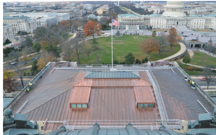
A view of the newly installed copper roof on the Jefferson Building's west main pavilion roof.
