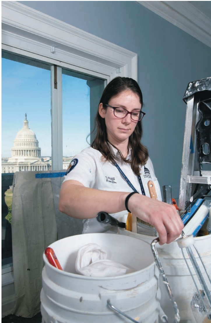
Donna Blake prepares the last coat of paint for walls located in the Jefferson Building's attic.
