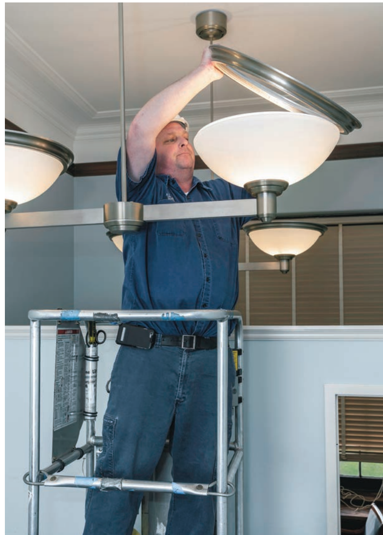
Brady Fleming, electrician leader with the Senate Electrical Branch, stands on a lift to adjust large lights in the Russell Building.
