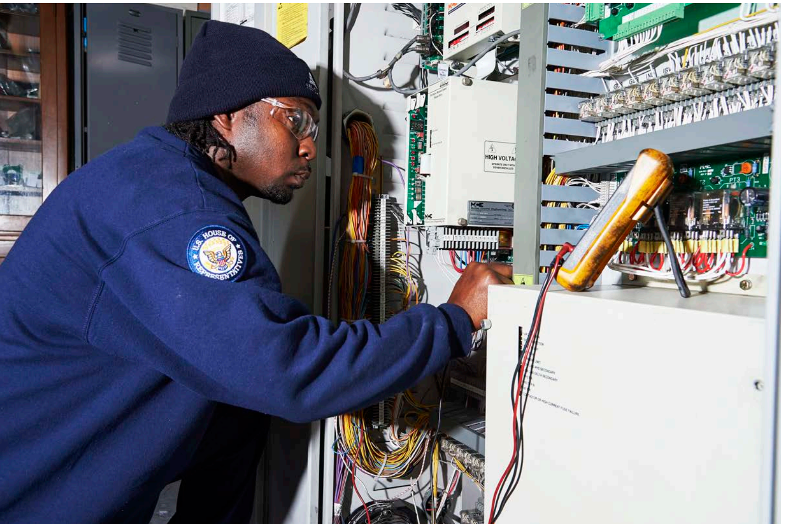
Alleyne uses a multimeter to diagnosis a problem with an elevator controller.
