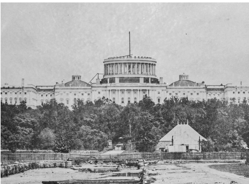
Dome construction from the West Front, showing the Dome skirt as a dark line below the Dome columns.
