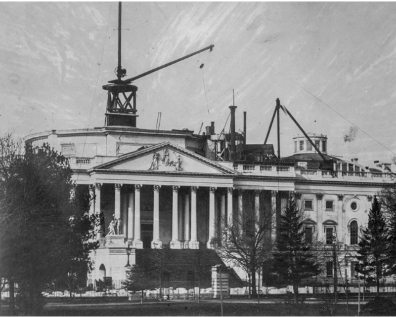
Dome construction from the East Front with the crane rising above the original sandstone Rotunda walls.
