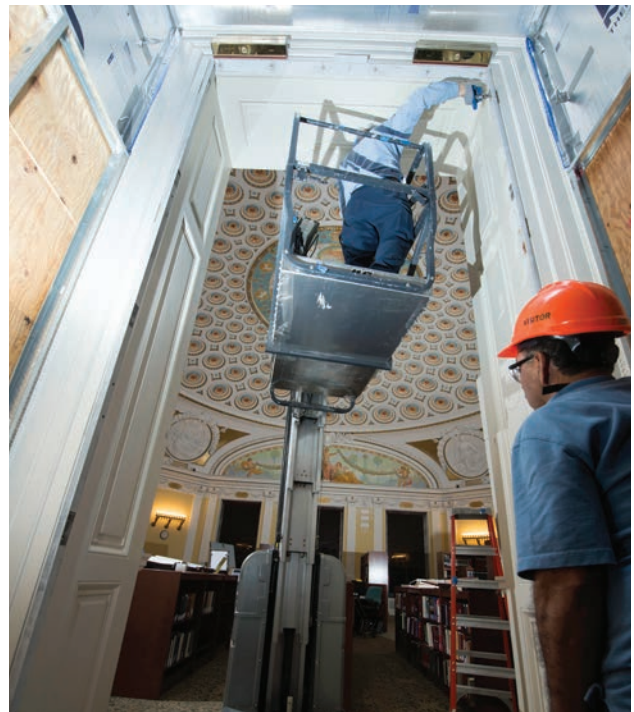
(left to right) Woodcrafters Bob Sheya and Jose Martinez were tasked with refitting new door hinge locations on existing door frames. The hinge locations on the doors were altered, and the existing locations were filled with wood shims.
