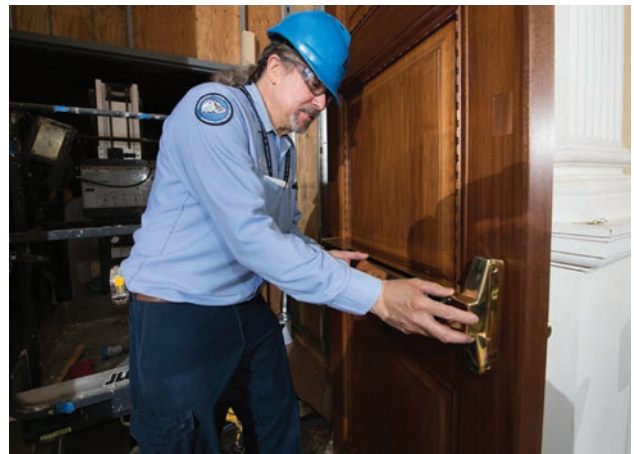
Bob Sheya installs new hardware as the finishing touch on a finished door. The entire process for one door from removing to re-installing and applying hardware was about two weeks.
