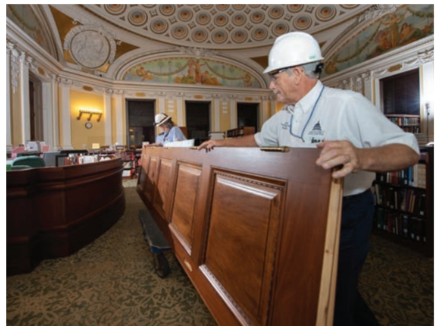
(left to right) Martin Jones and Nelson Samuels maneuver a door through occupied space on its way to being reinstalled. The pathways to and from the door locations had to be carefully planned to allow for the doors to be moved without damaging them or other items along the route.
