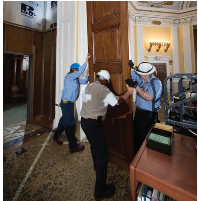
(left to right) Woodcrafters Bob Sheya, Nelson Samuels and Martin Jones carefully remove one of the 120-year-old historic doors, weighing upwards of 275 pounds.
