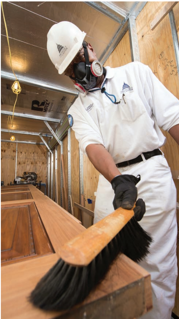
Painter/Re-finisher Darnell Johnson is shown prepping the door surface for stain after the old hinge locations were filled and sanded.
