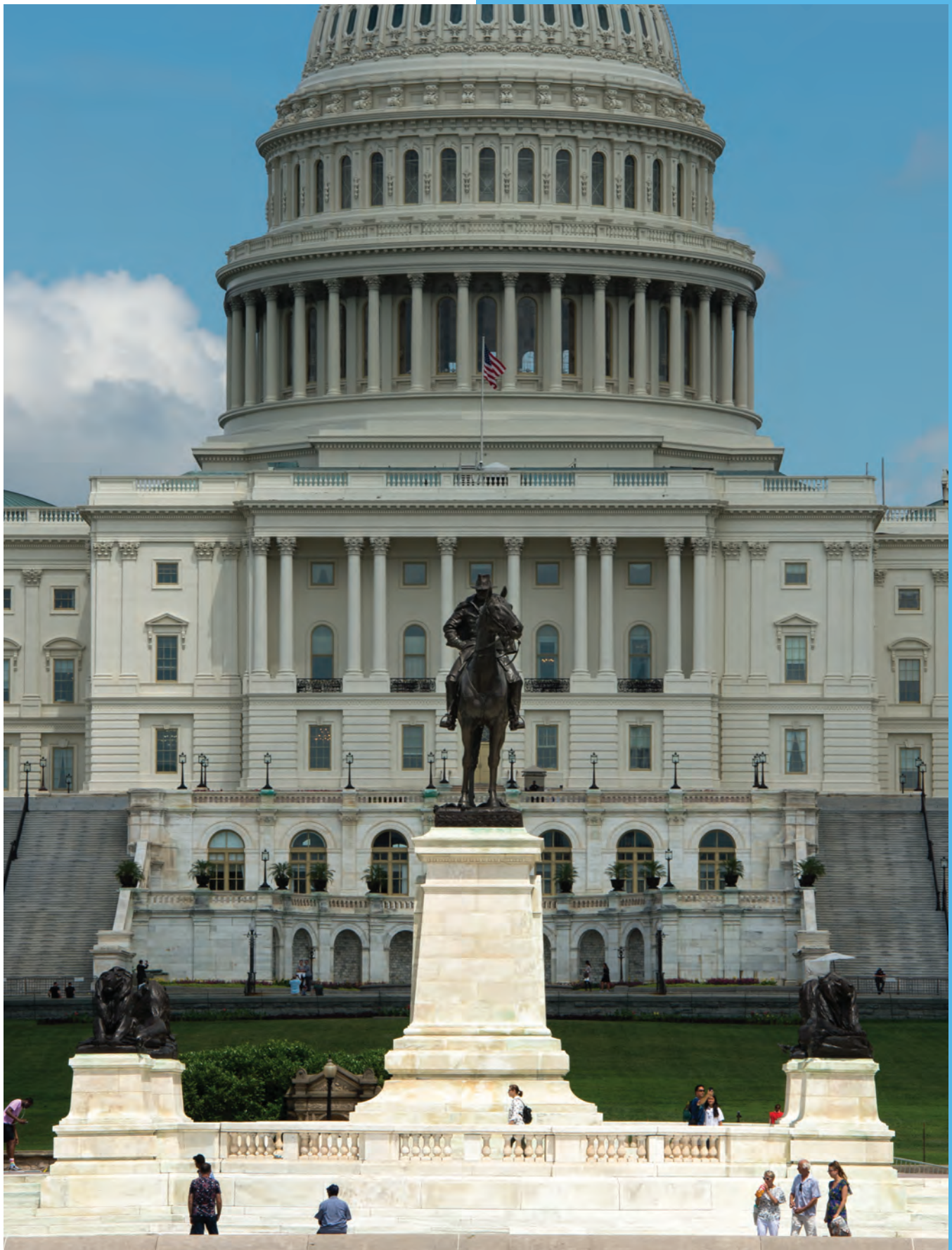
The Ulysses S. Grant Memorial has benefited from one of many stone repair projects the AOC is managing across the Capitol campus. In FY 2019, work on the Memorial's lower plaza began and was 80 percent complete at the close of the fiscal year.
