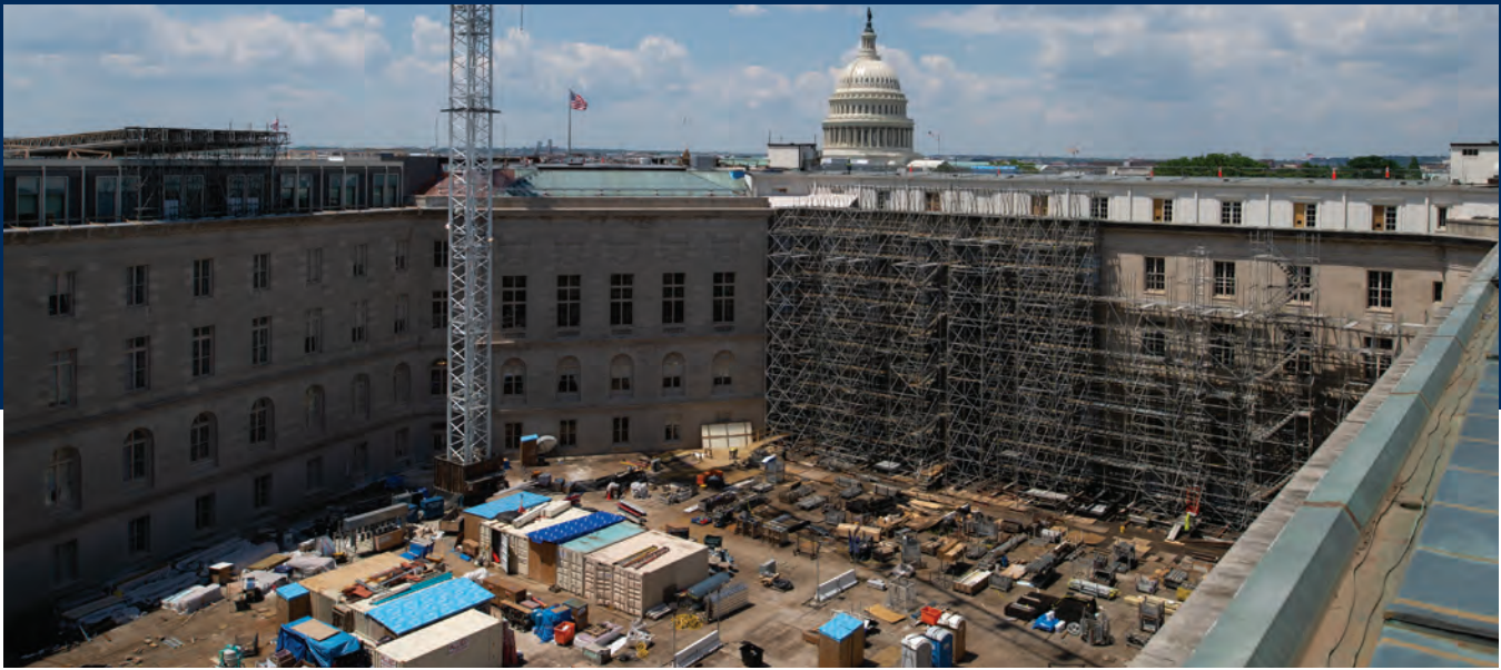
The Cannon Renewal Project, currently underway, will provide a comprehensive upgrade to the century-old Cannon House Office Building serving the U.S. House of Representatives.
