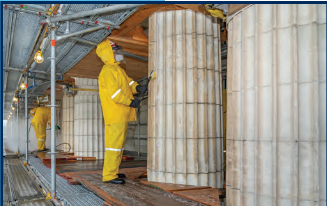
The AOC performed restoration work to the North Wall of the Russell Senate Office Building.
